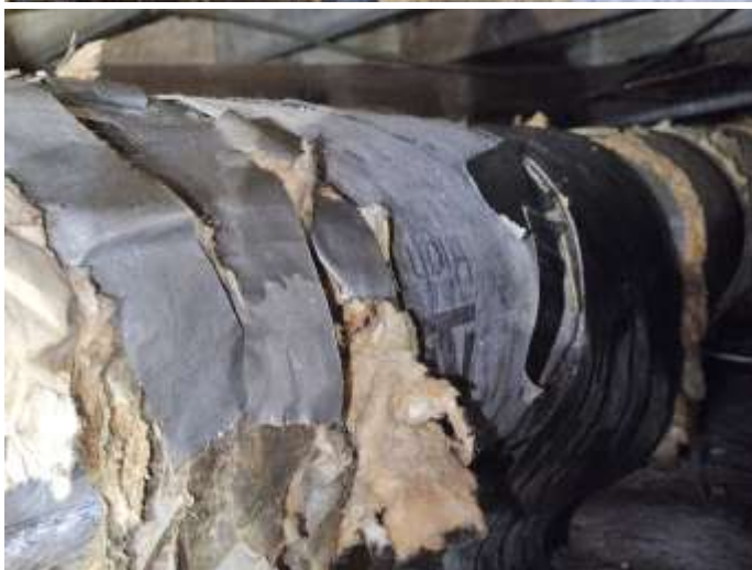
Duct system metal insulation deteriorating
