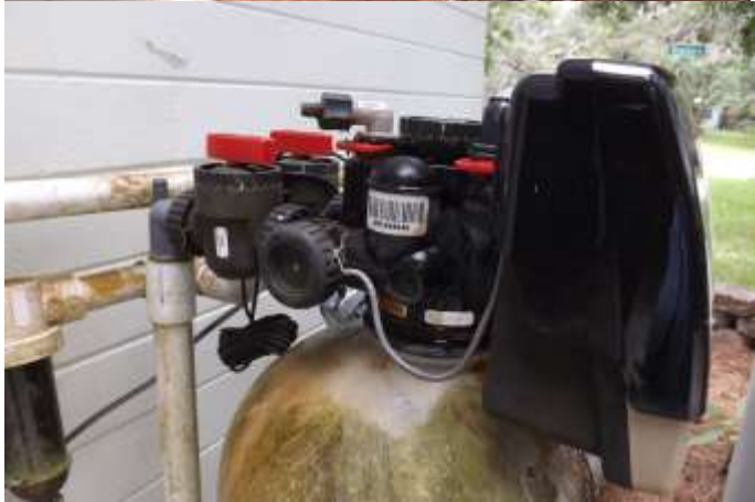
Water softener leak, Repair needed
