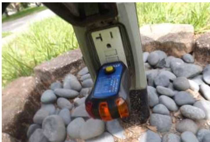
Front light pole outlet open ground GFCI protected
