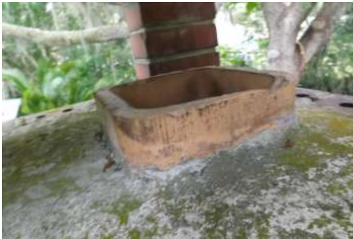
Chimney chips appear to be in good condition
