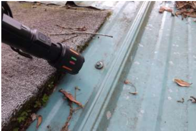
Roof screw installed in angle should be flat
