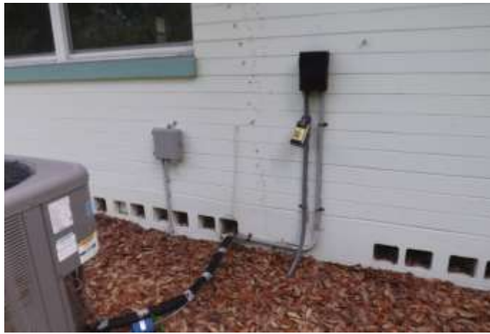
Can't find AC drain line
