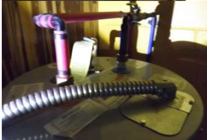
Water Pipe Copper & PEX
