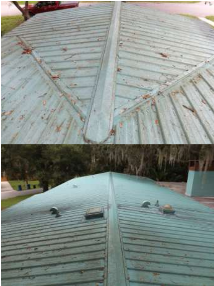
Skylights appears to be old or just very dirty from trees
