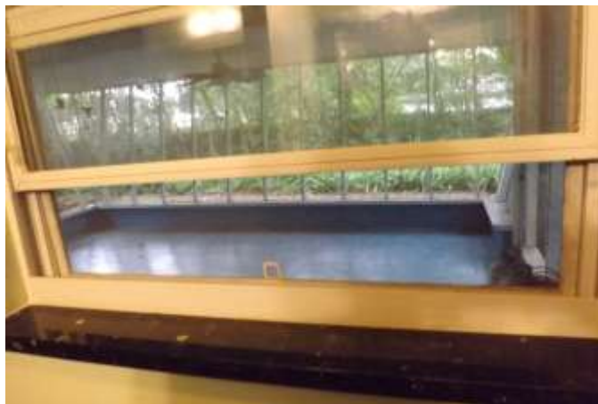
glass doesn't appear to be tamper replacement due to very dangerous
