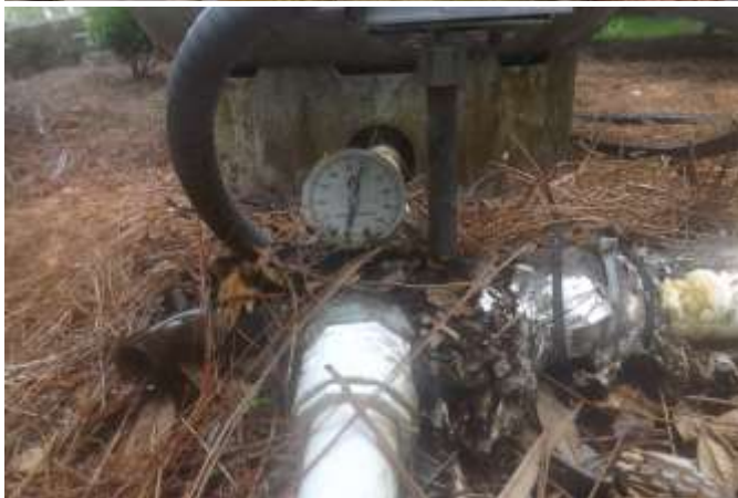
Gauge glass broken gauge appears to be working
