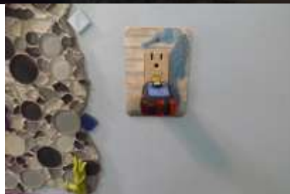
GFCI in good working condition
