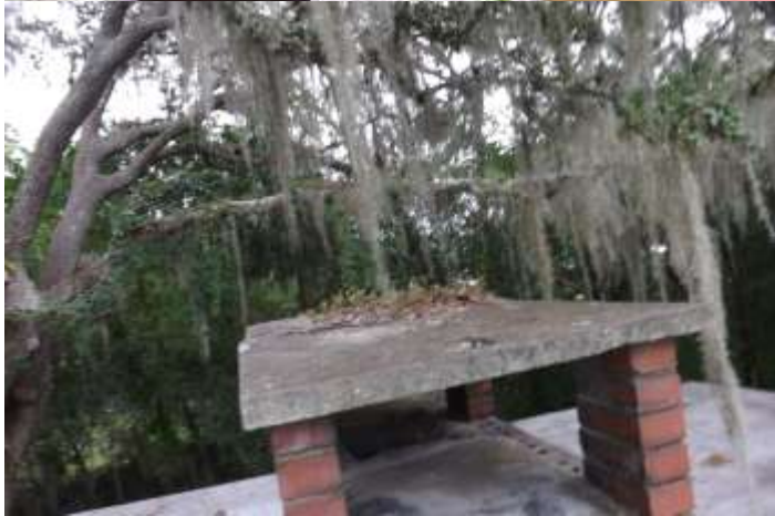
Chimney crown cleaning need & Seal cracks
