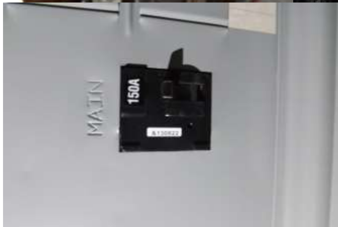
150 Amps Siemens Panel
