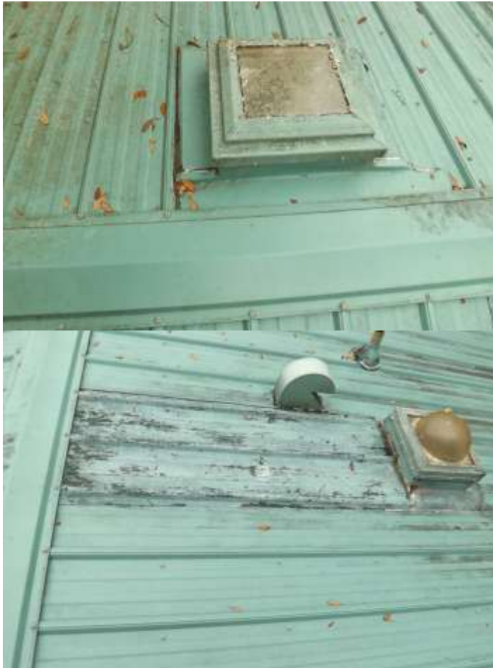
Roof panel appears to have been replaced or repairs
