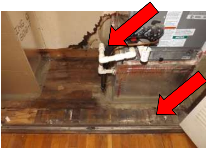
Air Handler leaking water damaged wall & floor
