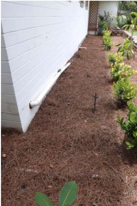
Washer drain going into ground not sure if hook
