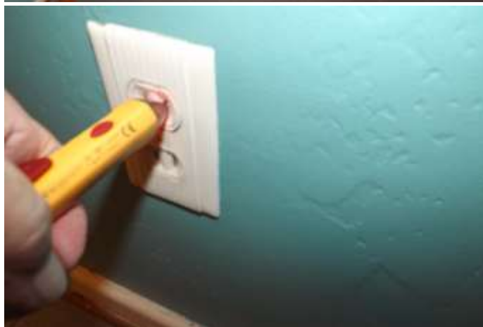
Outlet Open Ground GFCI Protected.
