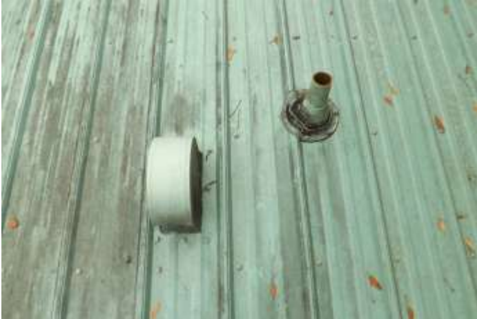
Waste vent Cast Iron
