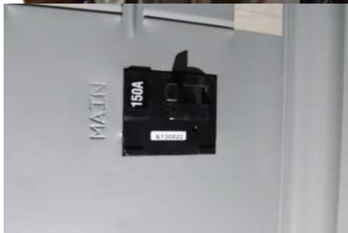
150 Amps Siemens Panel
