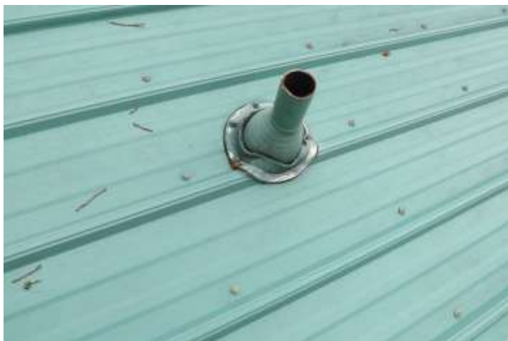
Waste vent cast Iron
