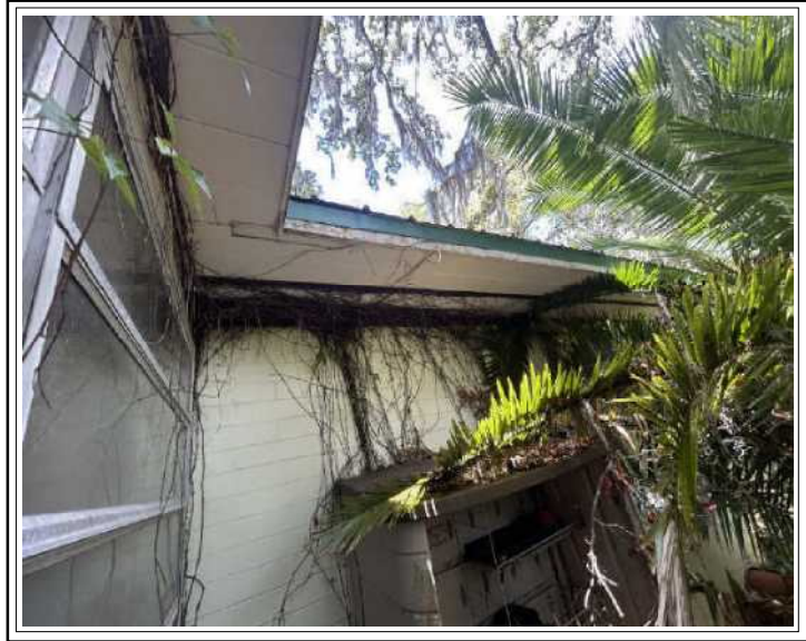
REMOVE DEBRIS / GROWTH
