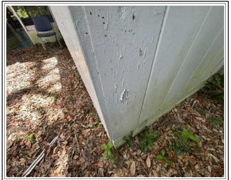
DEFECTIVE PAINT EXAMPLE
