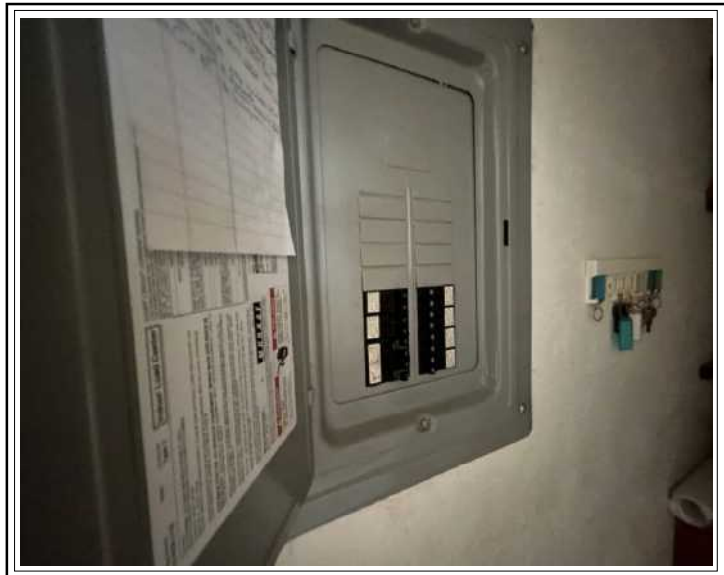
ELECTRICAL PANEL - NEWER
