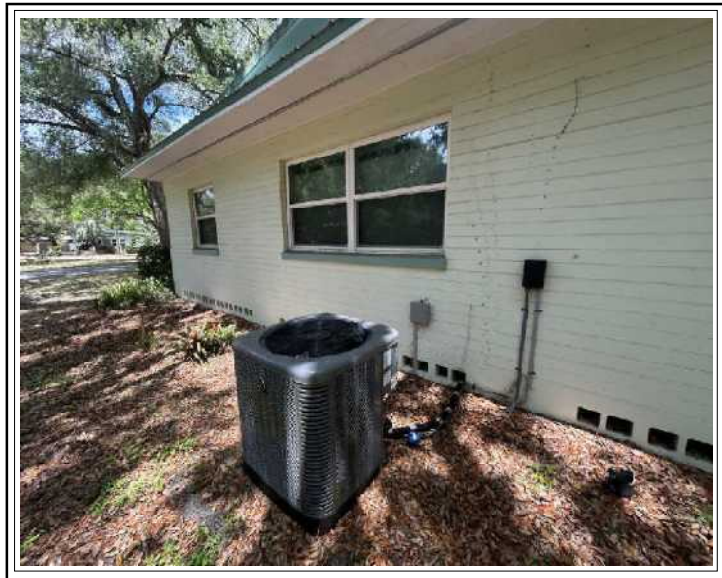
SIDE VIEW / HVAC
