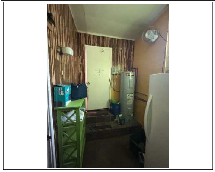
UTILITY ROOM VIEW 2 / WATER HEATER
