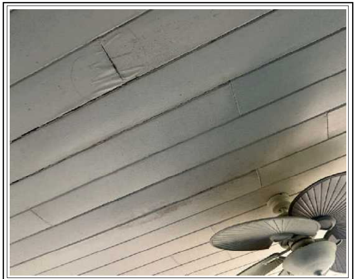
MINOR DECAY (FORMER LEAK - REPAIRED)
